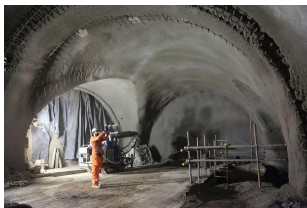
Figure 10. Site engineer using SMUTI to monitor shotcrete strength in the CONCI tunnel at Bond Street Station Upgrade
