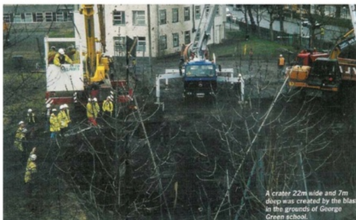
Figure 1: Blow out due to excessive compressed air pressure on the Docklands Light Railway Lewisham Extension on the 23rd February 1998 (NCE, 1998).
